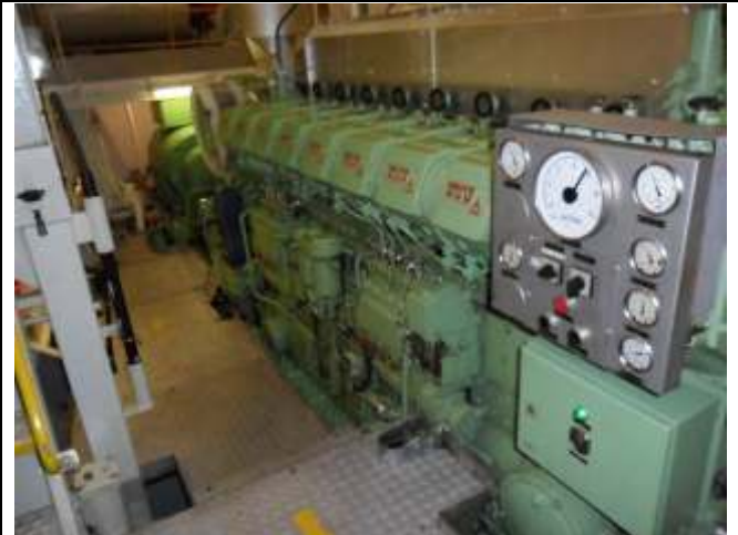
20. MAIN ENGINE FUEL PP PLATFORM
