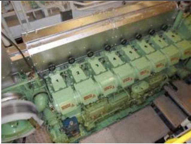
19. MAIN ENGINE CYLINDER HEADS PLATFORM
